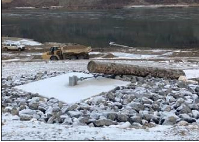
3 - Temporary Peace River Debris Boom Anchor (typical anchor)
